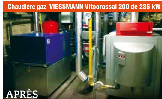
Chaudière gaz VISSMANN Vitocrossal 200 de 285 kW
